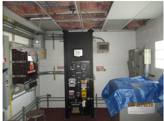
Here is a view looking inward from the door toward the inside of the NYMT substation. The large electrical panel in the center of the photograph was obtained during NYMT's earliest days and was formerly a part of a Denver trolleybus installation. Photo by C. Lowe.
