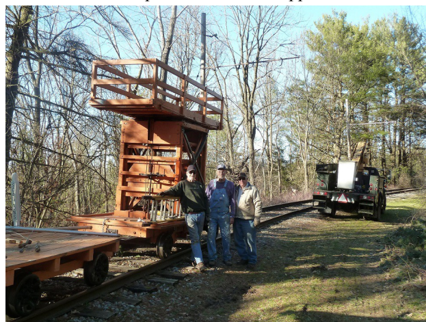
Line car 020 has been in use making overhead repairs. Here, from left to right, are Taylor Reed, Rick Holahan and Bob Achilles after an arduous day. In the background is one of the bracket arms just installed by the crew but before the contact wire was attached. In the background is the RGV bucket truck, generously made available to expedite repairs. Photo by C. Lowe.
