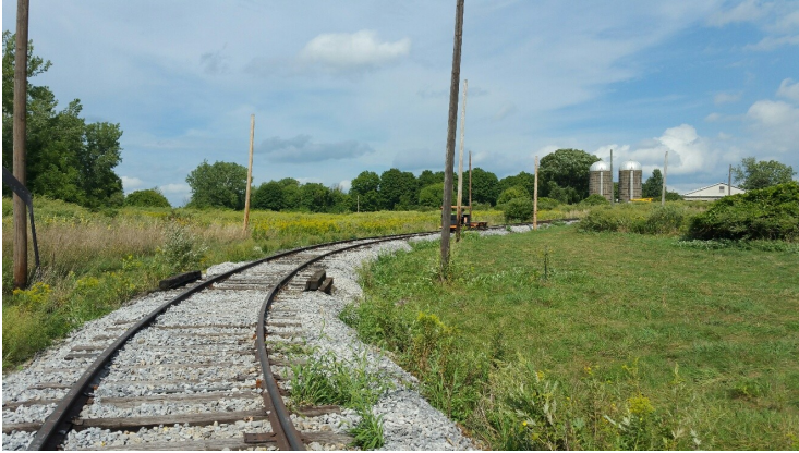
The east leg of the Loop Track has been transformed from an almost unusable section of the rail line to one which will soon host our trolley cars.
