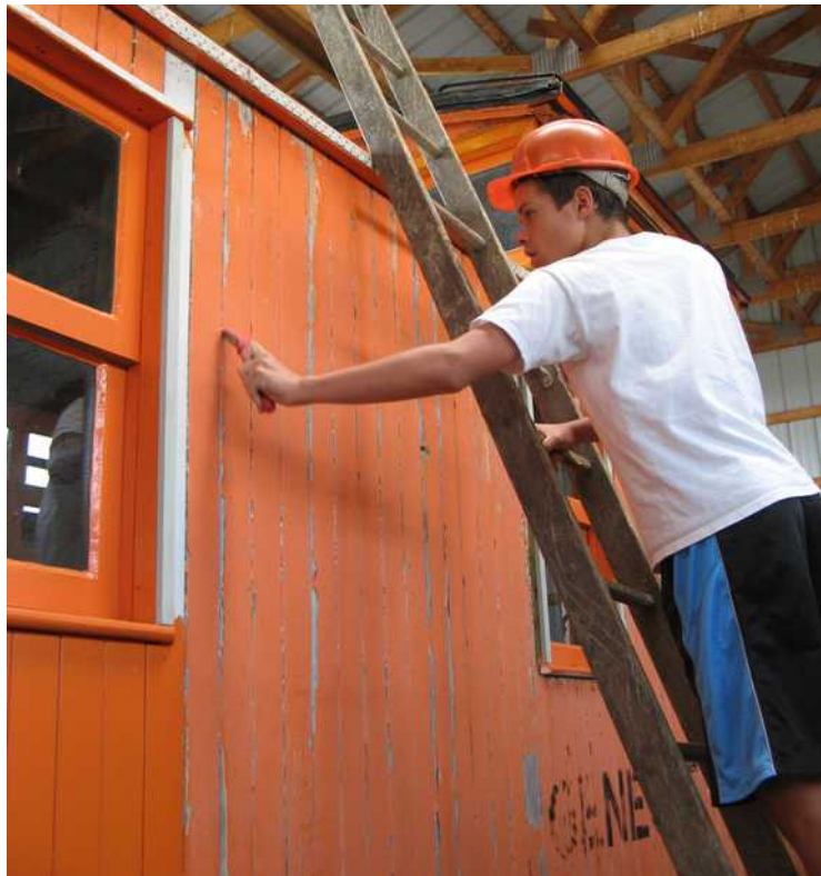
Justin Micillo is hard at work scraping loose paint from the side of the caboose, and modeling the G&W hard hat too.
